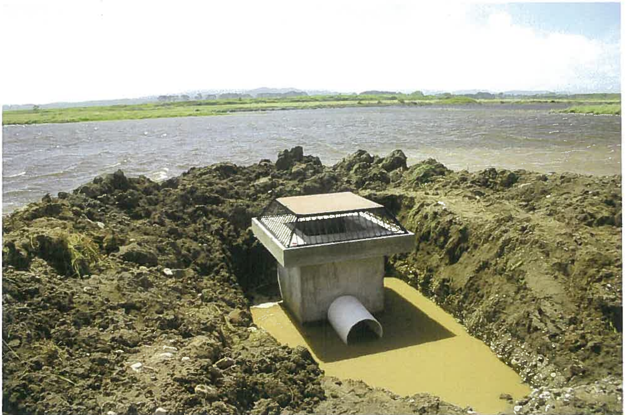
Whitebait Project. The installation of the siphon intake began in December 2015. The earth coffer dam protected the site from Inder wetland water inflows during installation.
