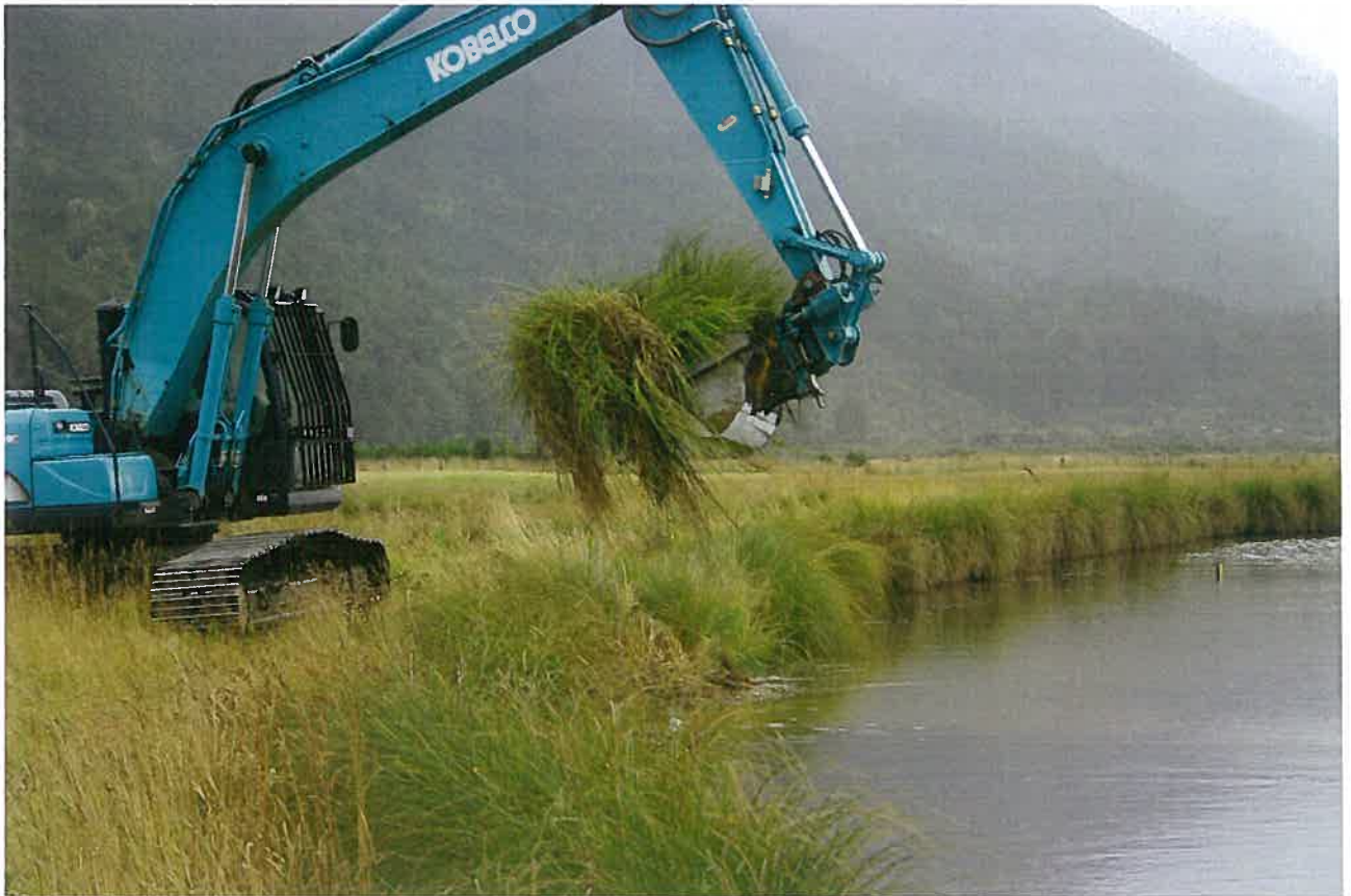
Rakatu Wetlands - dam face repairs, Speights Steam 2 wetland, March 2016. Wave lap action causing erosion along the north facing parts of this wetland was repaired by using existing vegetation from an adjacent wetland.
